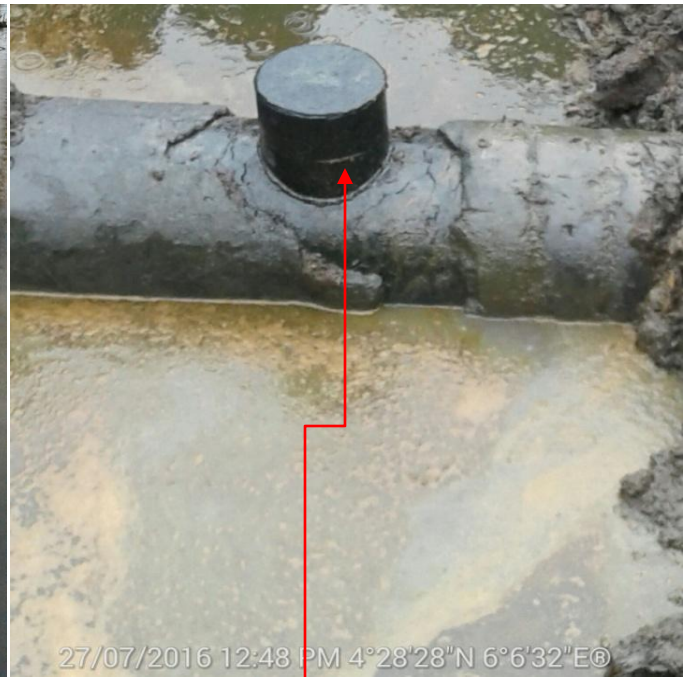
Fig B: The leak point (Hacksaw cut)
